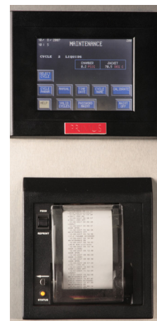
Trinity Control Panel with Thermal Printer
